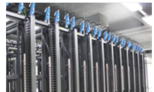
Internet Data Center, South Korea
