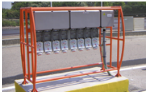
Container Terminal, Le Havre, France
